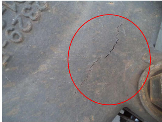
Figure 8 - Manway cover top side cracked
