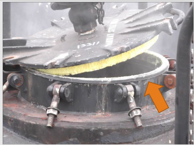
Figure 12 - Manway nozzle gasket
