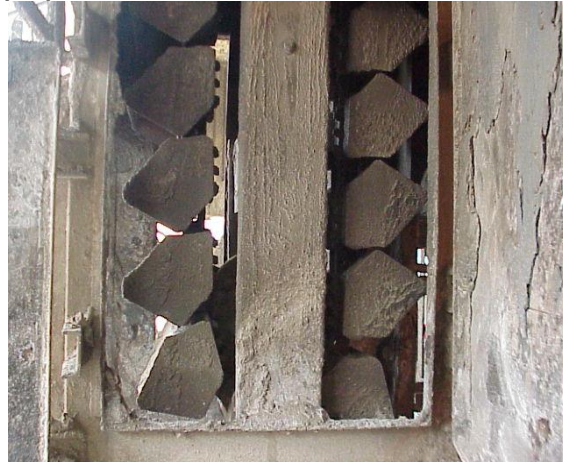
Bucket Elevator – Becomes a confined space when the buckets are removed.
