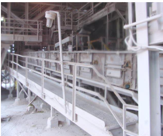
Drag Flight Conveyor – Becomes a confined space when the drag flight is removed.
