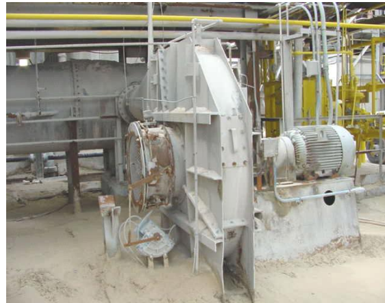
Small Blower – This is not a Confined Space
