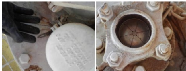
Figure 15 - Inspect Rupture Disc
