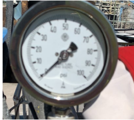
Figure 29 - Check pressure gauge
