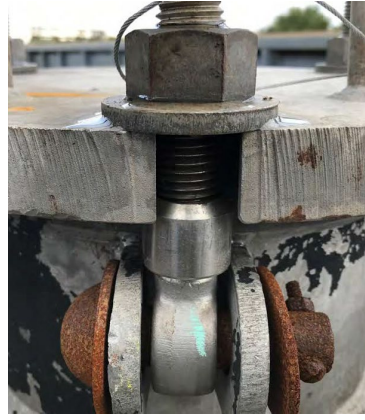
Figure 19 - Safety eyebolt out of adjustment. Bad order car, do not ship
