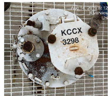
Figure 13 – Top fittings with no protective housing
